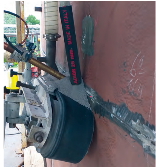
Fig. 6 — DSAW carriage and flux support system.
